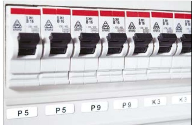
Clear and permanent identification of switch gears.
