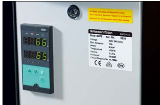
Professional type plate on a heating unit.
